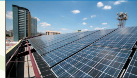
Above: Photovoltaic panels were incorporated into the design of the Pennington Street garage in Tucson, Arizona. These panels supplement the facility's electrical system by providing 50KW of electricity and are tied directly into the City's power grid on the roof.
